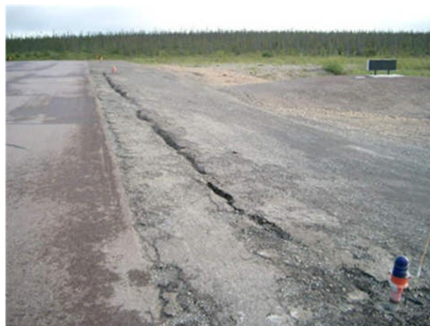
Longitudinal cracks along embankment shoulder, Forward Operating Location (FOL) Inuvik. Photo credit: Lance Gelin, DND, from: Tunnicliffe and Burn, Towards a Protocol for Airport Infrastructure Risk
