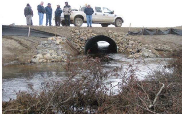
A tour of a new section of highway near Inuvik highlights a sagging culvert – issues that will have to be addressed in new roadway design. (photo from Jun 9, 2011 site tour documentation; EBA Engineering).
