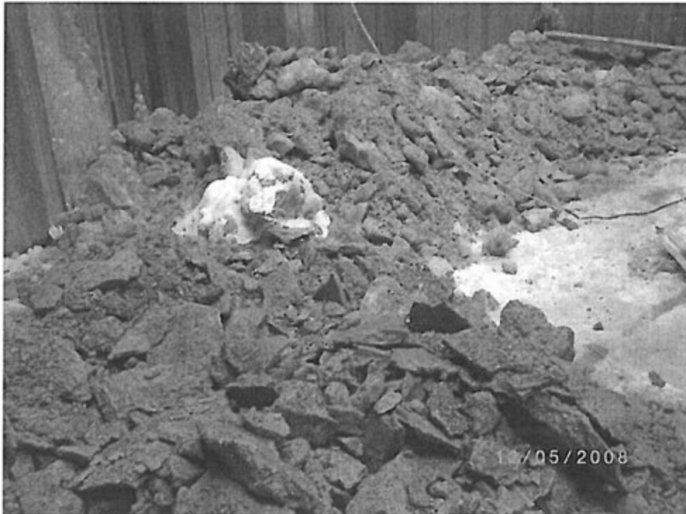
Photo 4: Debris piled against cofferdam, December 12, 2008.
