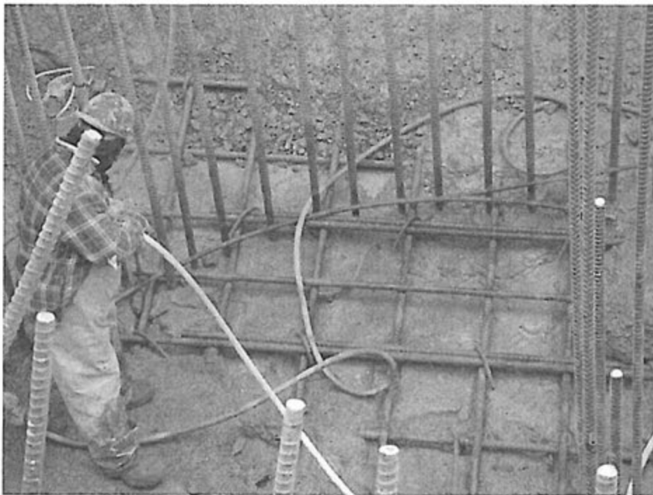
Photo 3: Close up of area shown in Photo 2.
