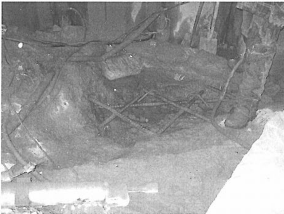
Photo 6: Depression near cofferdam, November 12, 2008.
