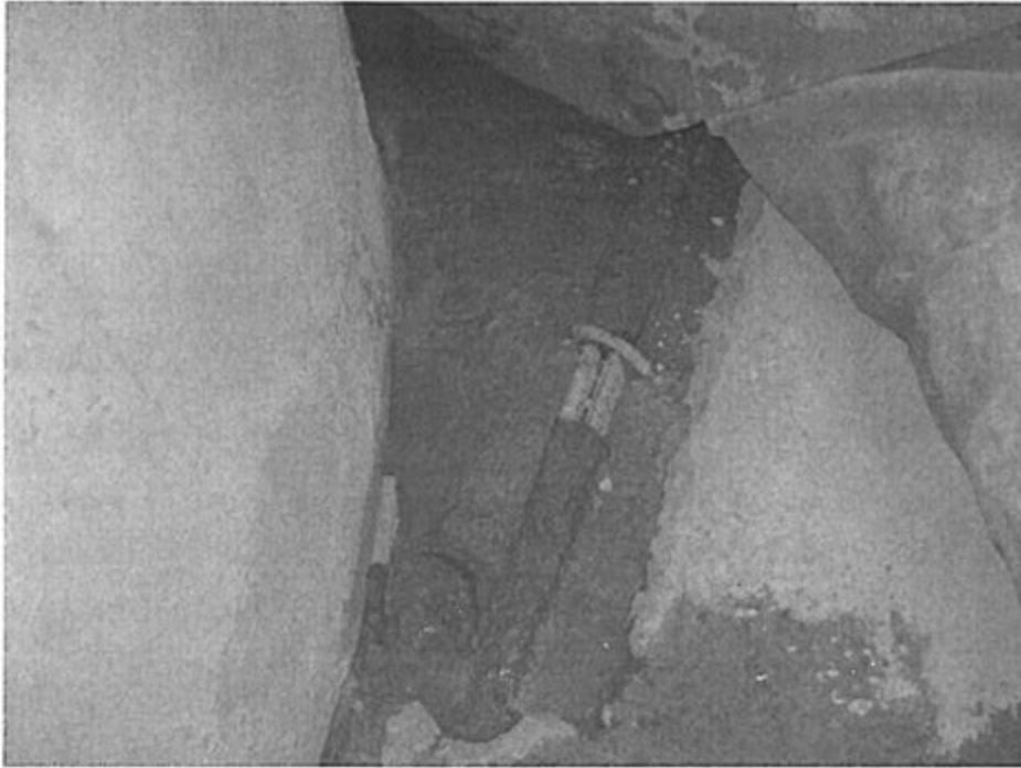
Photo 5: Depression partially filled with fresh concrete, November 7, 2008. This appears to be the same area shown in Photo 1.
